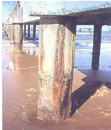
Characteristic attack due to corrosion of reinforcing walkway structures in the intertidal zone
