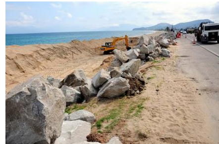
SP-55 Highway that connects Caragutatuba to Ubatuba. Work protection embankment to correct erosion and minimize flooding
